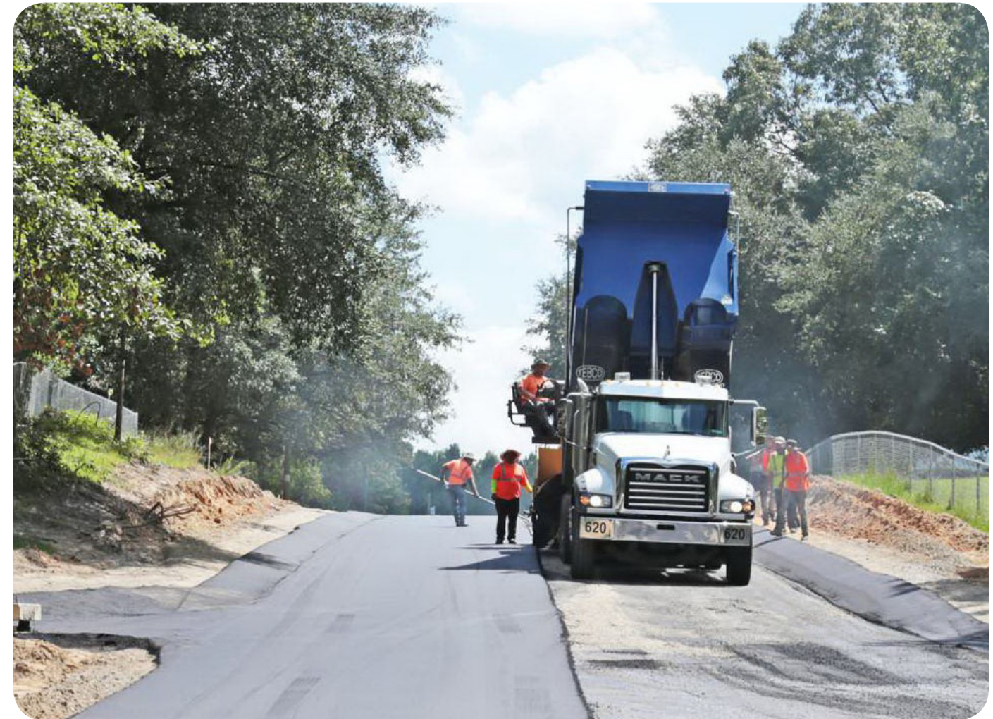
Photo: Road Paving on Peacock Dr. Funded by Sumter County Capital Projects Sales Tax
